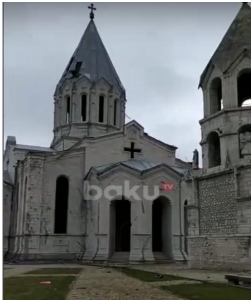
Image 5: The shelled part of the dome of the Holy Saviour Ghazanchetsots Cathedral as of December 11, 2020
